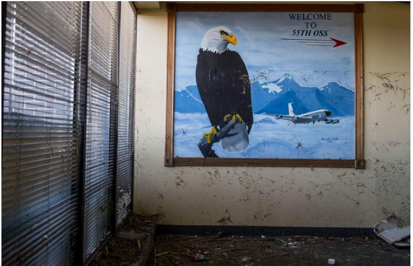
Debris indicates the high-water mark left by March flooding in the 55th Wing Headquarters building at Offutt Air Force Base.
